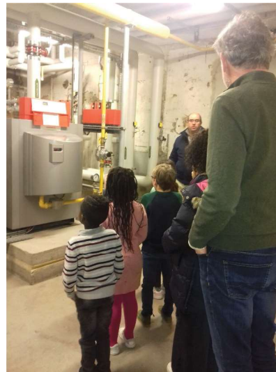
Visite chaufferie (Clermont)
