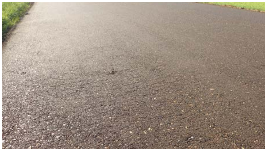
Figure 5 / ORRAP Switzerland - Vibration that can generate cracks. Source Cerema
