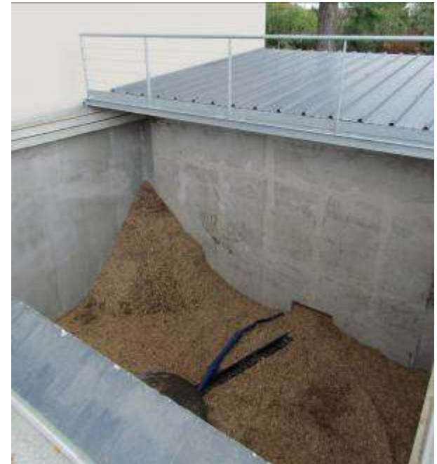
Chaufferie Bois - St Varent
