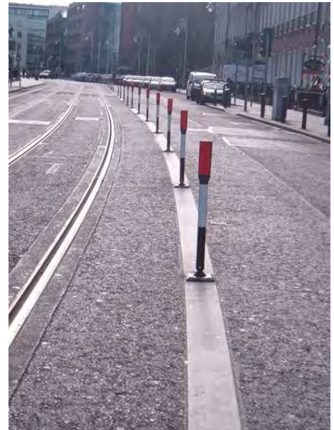
Figure 135 – Dublin, Plastic bollards along the white line demarcating the swept path of the tramway
