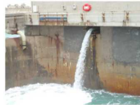
Station de pompage
