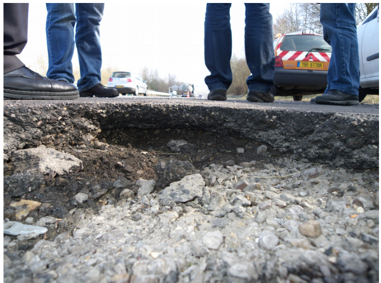
Dégradation of surface course – Photo Cerema
