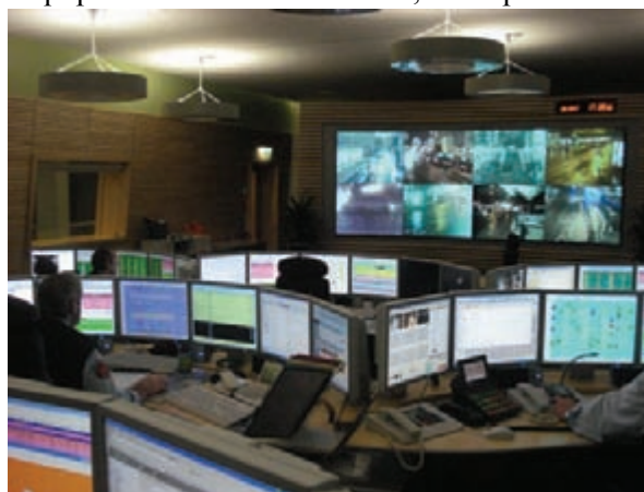
AVM Control Centre of PT Hamburg, for all lines on surface
