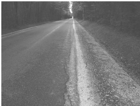
Illustration 38: crack on the side ("beam" effect of the concrete wall)
