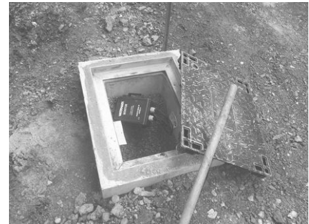
Illustration 34: Recording box in a manhole under the shoulder
