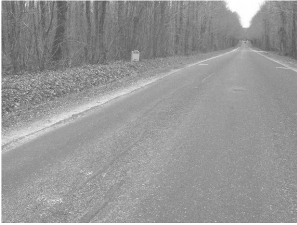
Illustration 40: state of the location at PR5 in January 2015 (3 years after confinement works)
