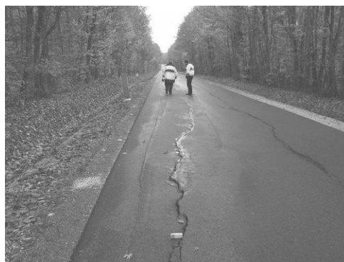
Illustration 27: longitudinal cracking (adaptation cracking)
