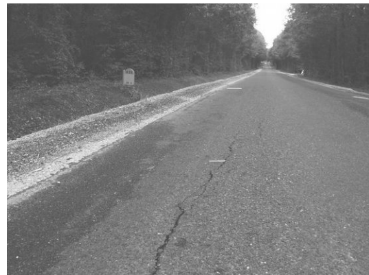
Illustration 39: longitudinal cracking with edge settlement (same place as illustration 27)
